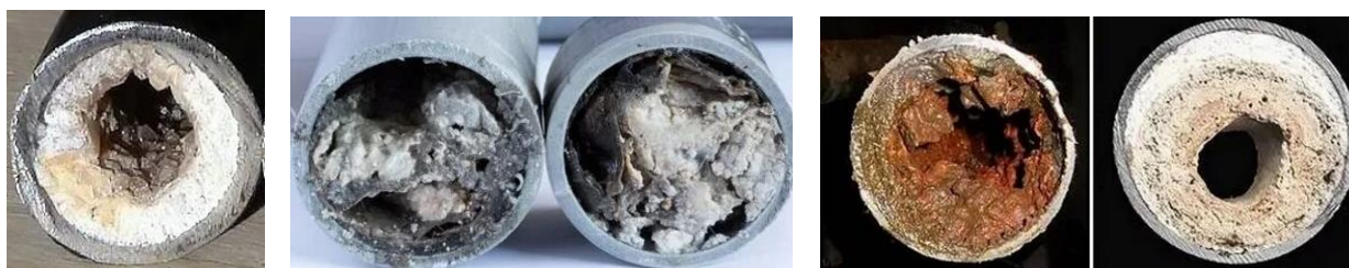
Figure 1. Partially or completely clogged sewer pipes [1-5]
